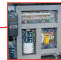
ACCESSIBILITY Easy access to electrics if required
